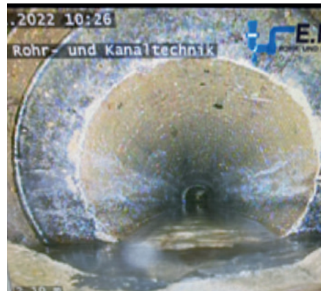
Axial displacement visible in an underground pipe
